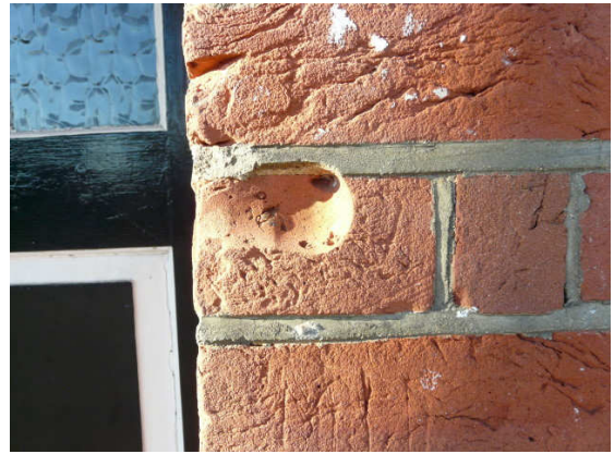
21. Village Hall Porch – wear due to handle – K4:
